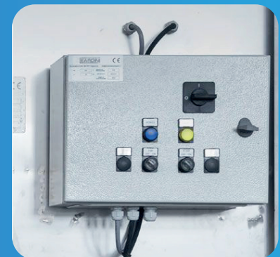
Panel de control
