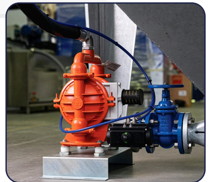
Sludge suction pump: Extracts the settled solids after decantation and sends them to the compaction system.
