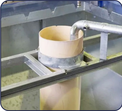
Dirty water inlet pipe.
